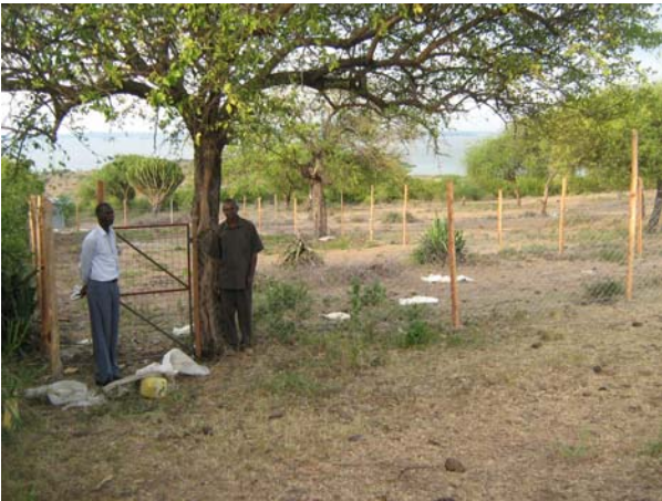
With a new fence, work on the school garden can now begin
